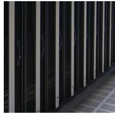
Data Centre Ventilation
